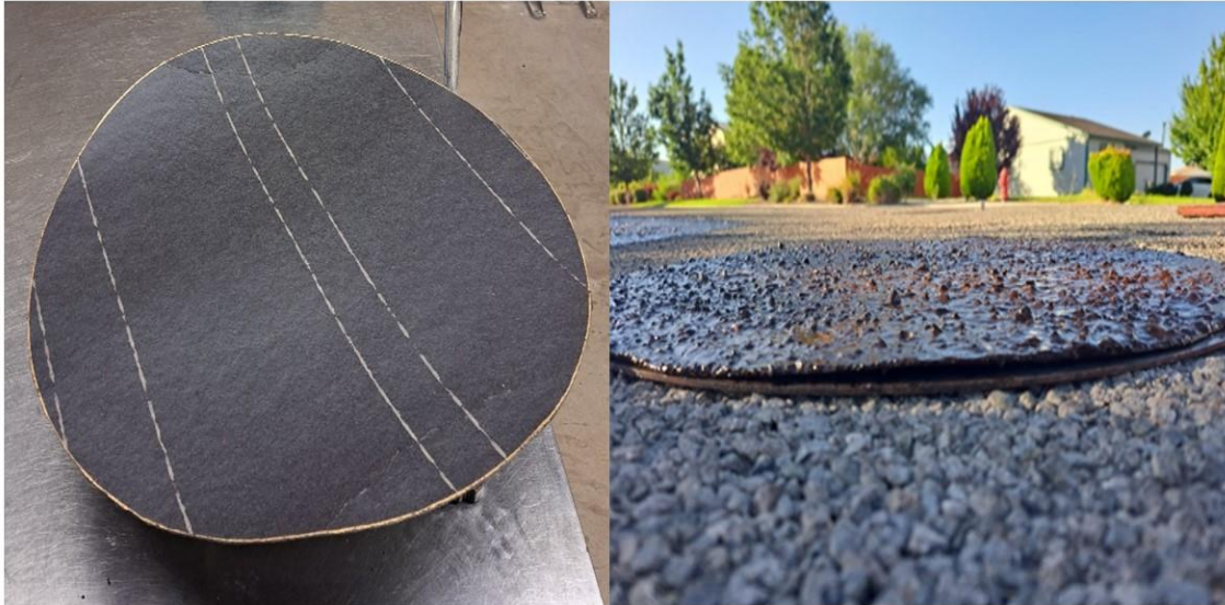
Figure 3. Asphalt felt was used over the utility cover to collect slurry mix samples.
