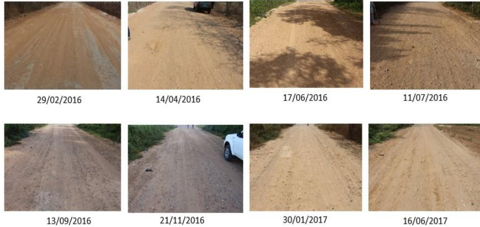
Figure 11. Deterioration evolution in the BD track.
