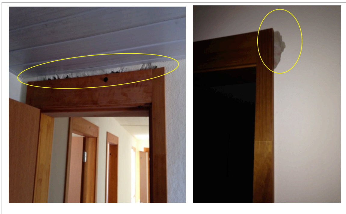
Figure 3. Examples of problems in the interface between the wood flashings and plaster. Source: authors
