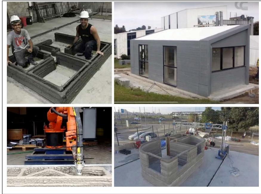
Figure 3. 3D printed construction experiences in Latin America and Spain (top left: 3D housing construction, Brazil; top right: Conconcreto, Colombia; below left: HausDrucker, Argentina; below right: Be More 3D, Spain). Source: the following websites: ( https://www.facebook.com/pages/3D-Home-Construction https://conconcreto.com/impresora-3d/ https://www.youtube.com/watch?v=ASTwjgs7jKw , https://bemore3d.com/ )
